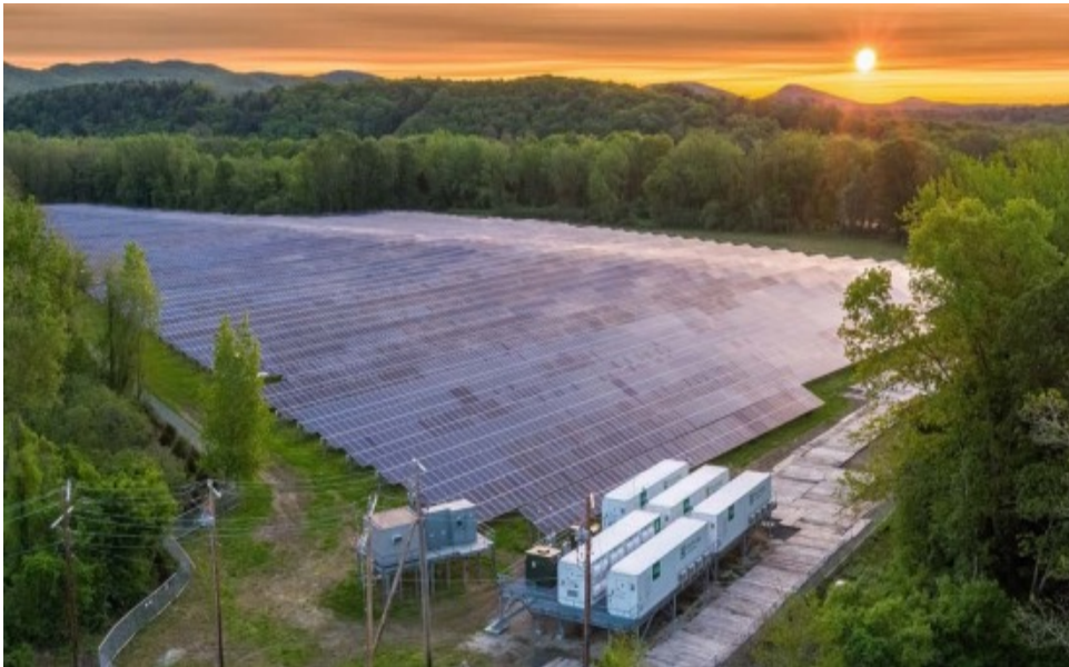
Distributed solar-plus-storage project in Holyoke, MA
