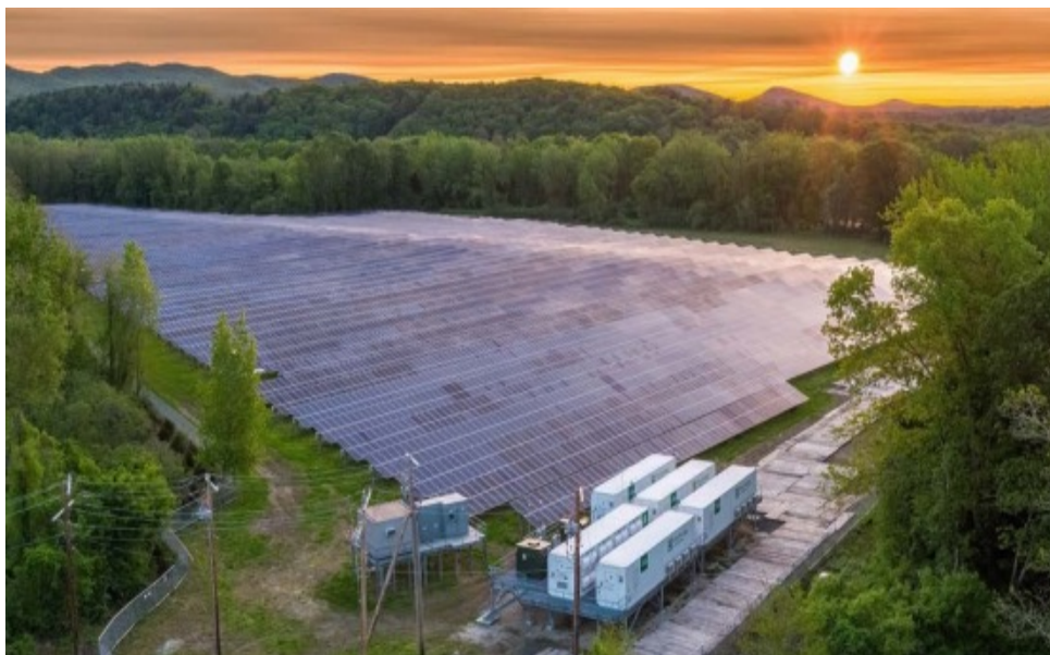
Distributed solar-plus-storage project in Holyoke, MA
