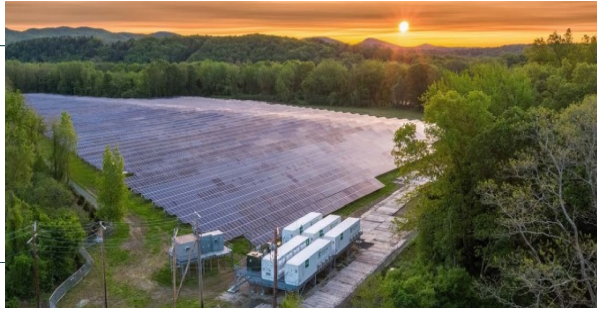
Distributed solar-plus-storage project in Holyoke, MA
